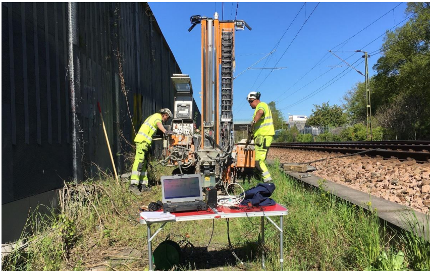
Figure 2. Measurement setup of soil-rock sounding (background) in combination with vibration measurements (foreground).
